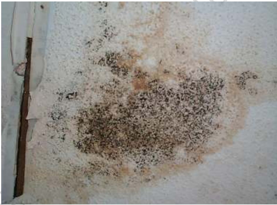
Black mold on gypsum board
